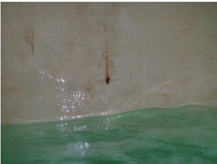
38) A few spot coating breaks were found on the sidewall above the high water level.
