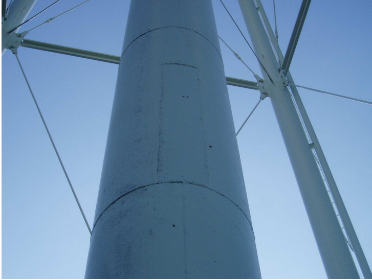
16) Another view of the exterior riser with spot failures.
