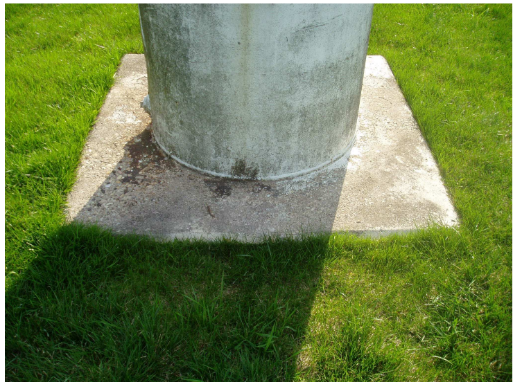
5) Mildew growth on the bottom of the exterior riser.
