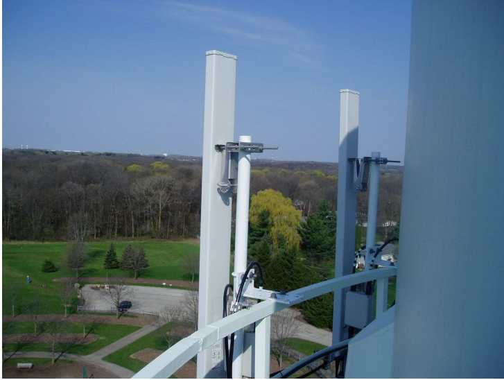
22)Antennas mounted to balcony handrail.
