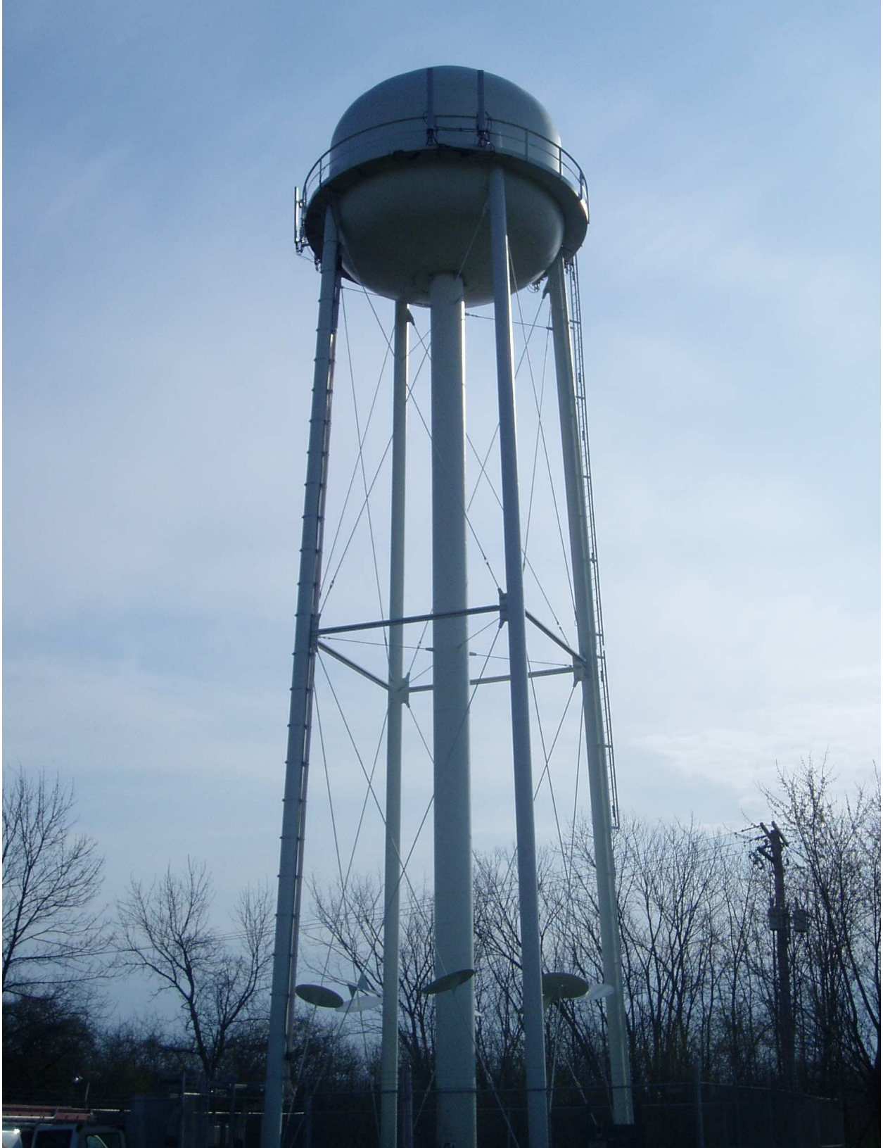
Looking at the 40,000 gallon legged tank owned by Lake County DPW.
