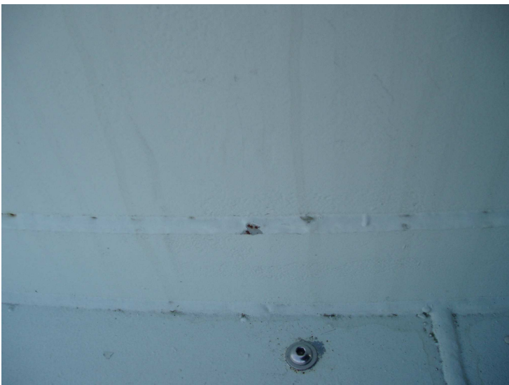
24)Coating delamination on the lower exterior sidewall.
