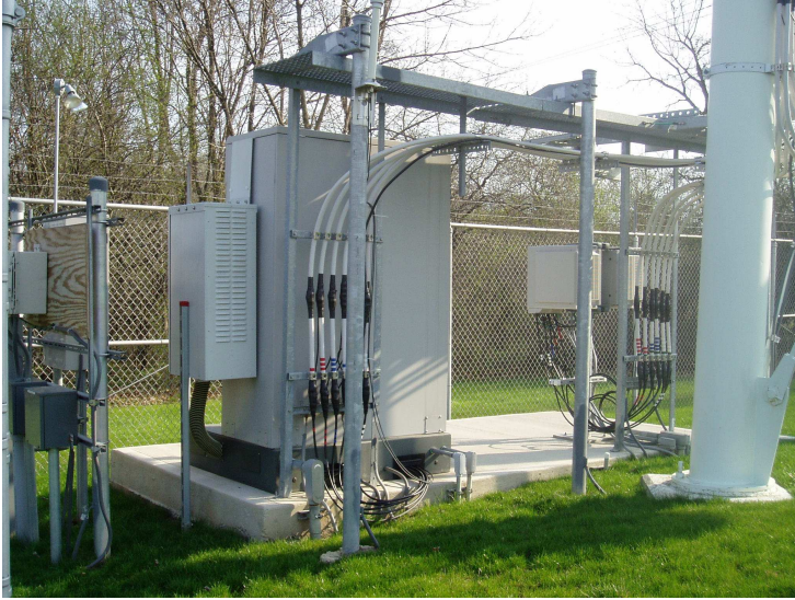
4) Antenna equipment located next tank leg.
