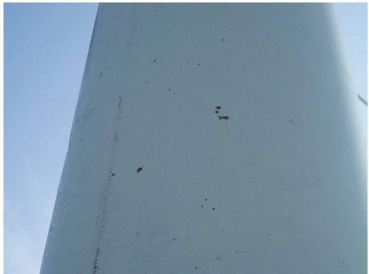
8) Spot coating failures on the exterior riser.
