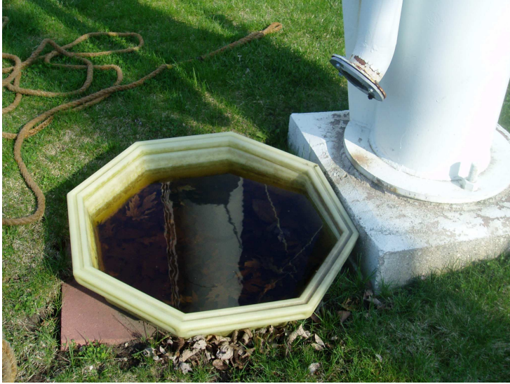
13) Overflow pipe with discharge area.
