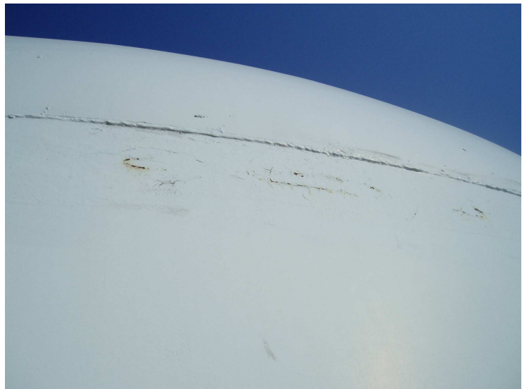
25) Coating damage to roof coating from ladder wheels.
