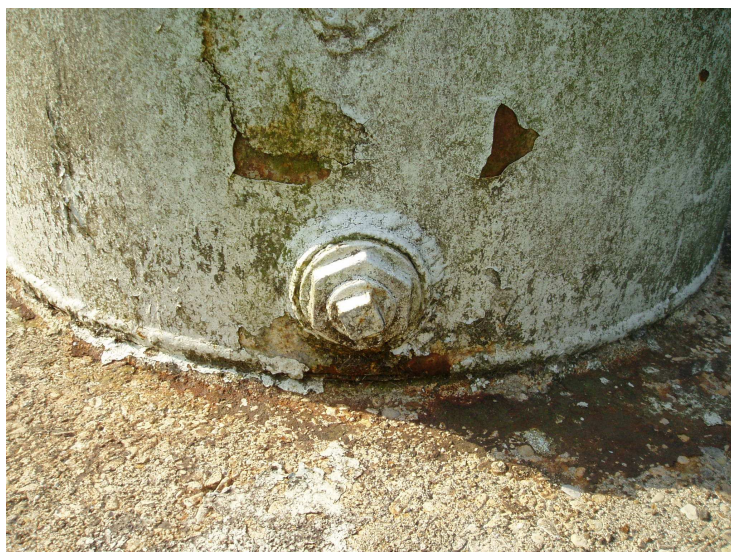
6) Coating delamination on the bottom of the exterior riser.
