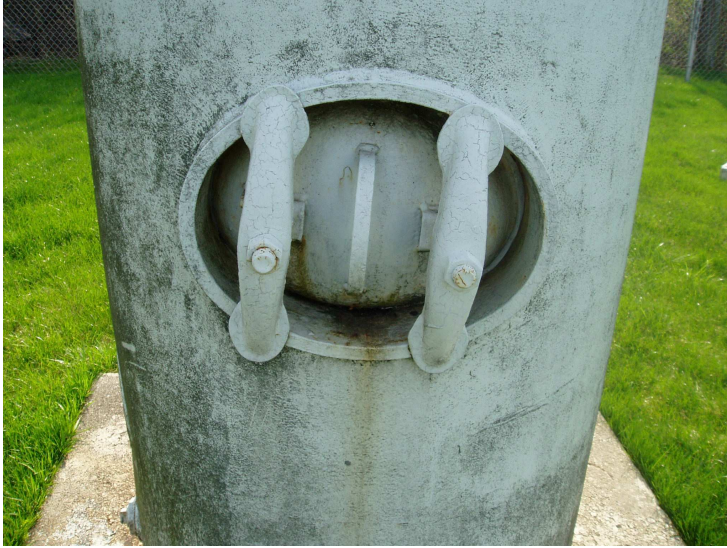
7) Bolted manway at the bottom of the riser.
