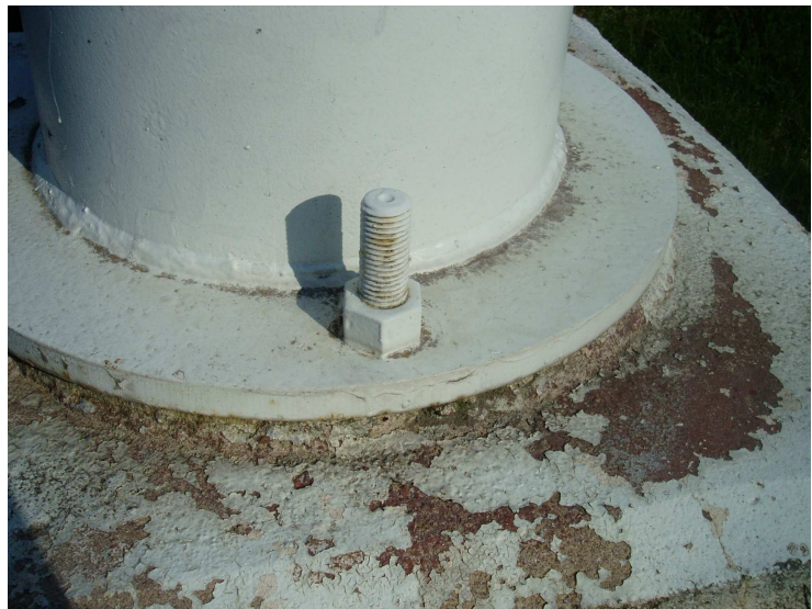
11) Area of missing grout between leg base plate and foundation.
