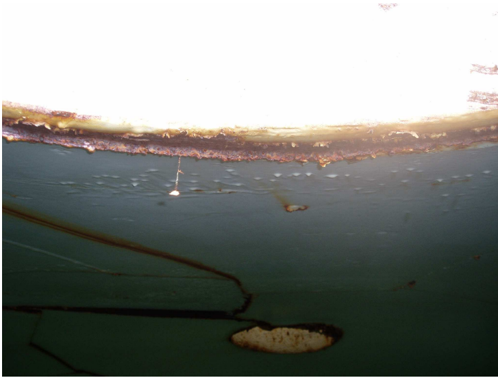
33) Rusting is occurring on the edges and in the crevices of the wet interior roof.
