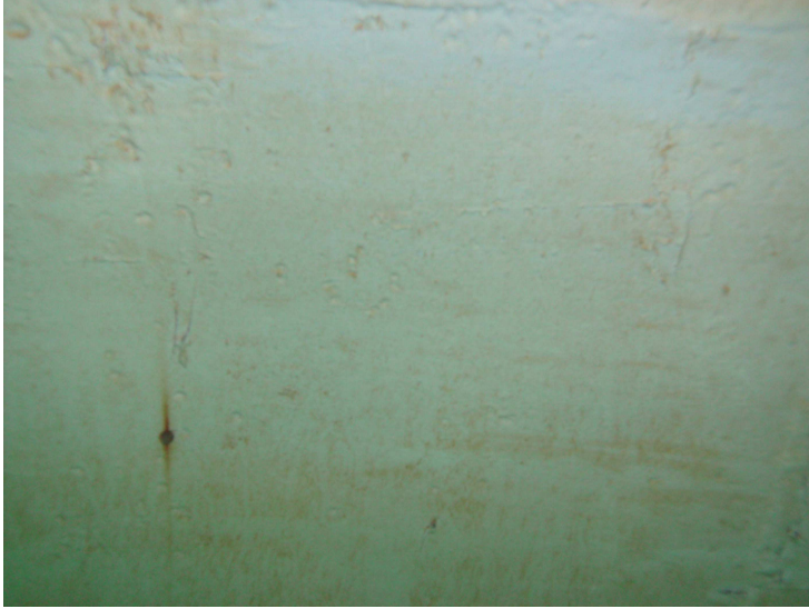
39) Spot coating breaks were found on the sidewalls below the water level.
