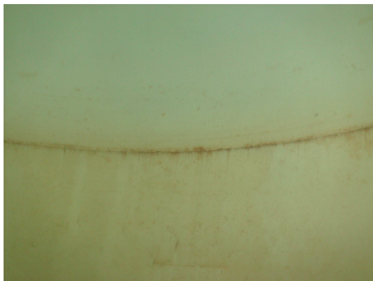
41) Coating on the sidewalls below the water level is in good condition.
