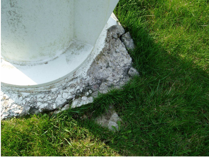
10) Leg foundation is has large areas of spalling concrete.
