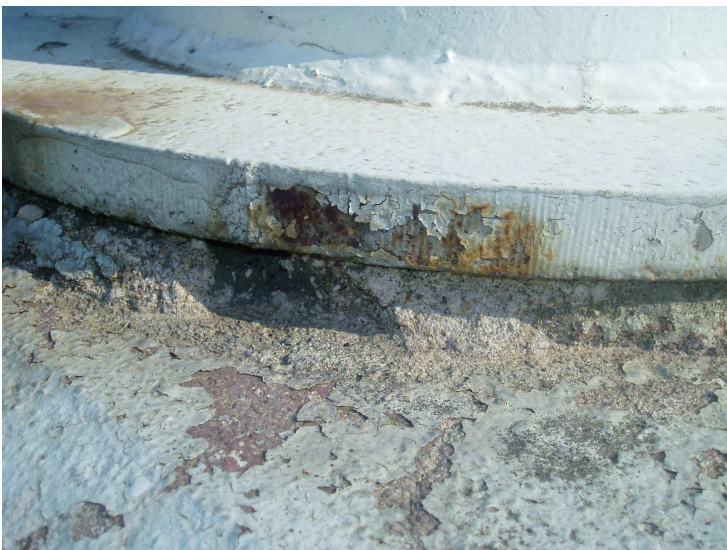
12) Closer view of the missing grout.
