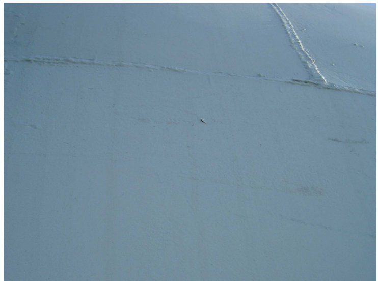
23)Spot coating failures in the exterior sidewall coating.
