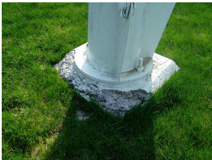
9) Foundation for an exterior leg is in poor condition.
