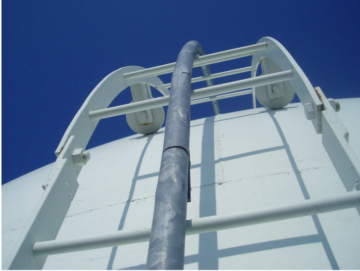
24) Revolving roof ladder with rail fall prevention.
