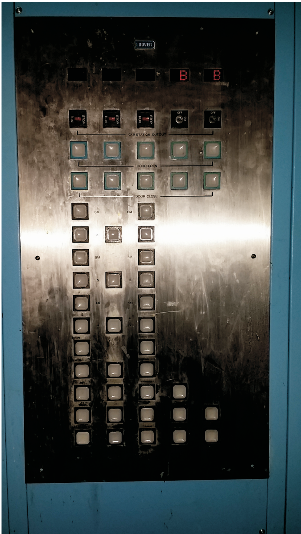
Jail Base Bid Item # 1.0 and Bid Alternate Item 4.0 Remote Control Panel for Central Control Operations. The Fire Alarm Panel is also located in the same area
