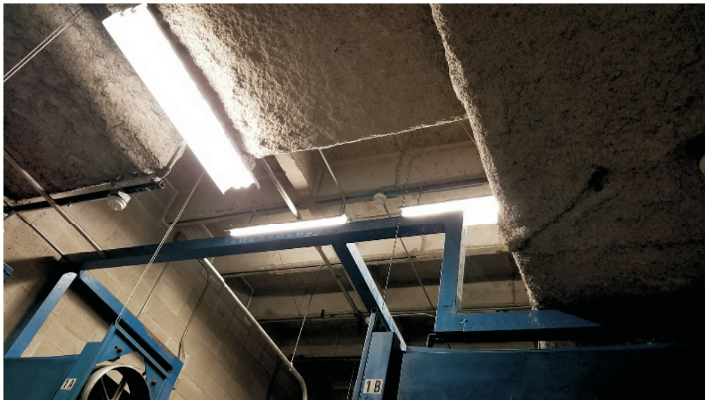
Elevator Machine Room Ceiling Pic #1
