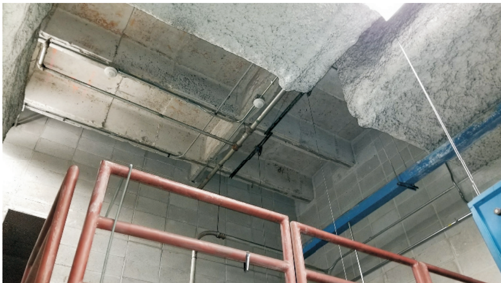
Elevator Machine Room Ceiling Pic #2
