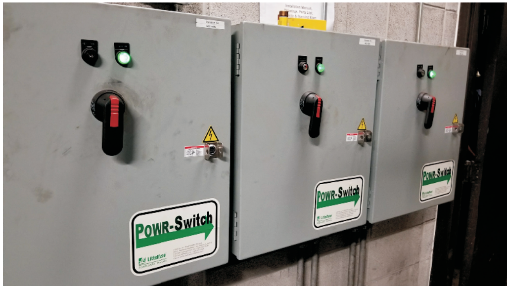
Elevator Shunt Trip Disconnects with Fire Alarm monitoring
