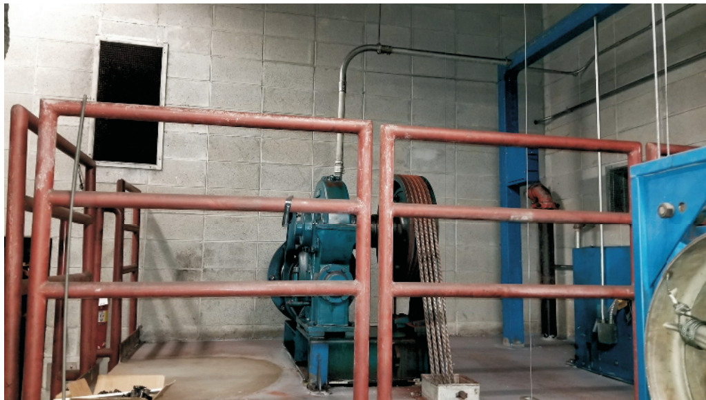
Jail Visitors Elevator Motors, pulley and brake Bid Item #4.0
